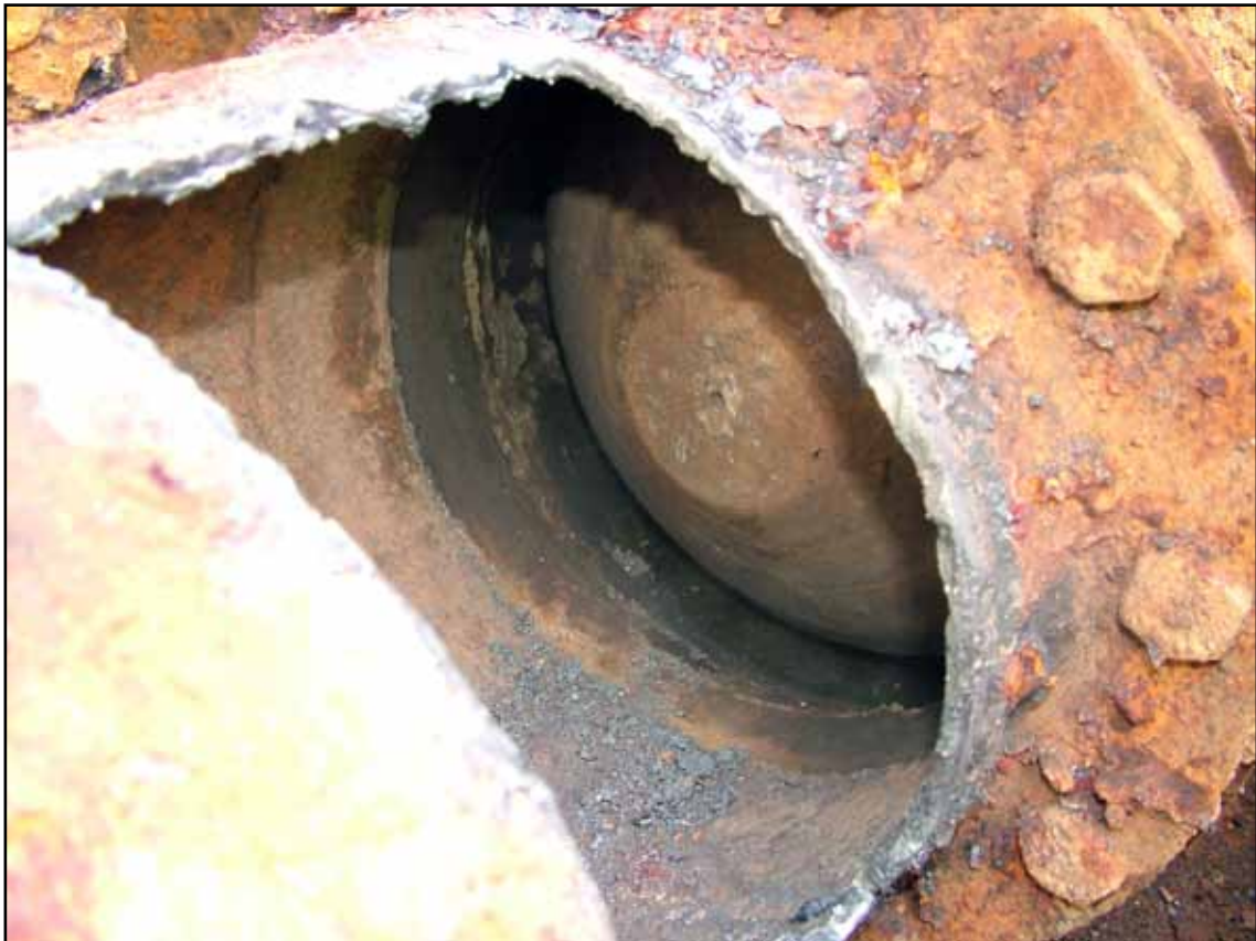
Port non return valve not sealed
